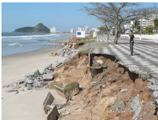
Coastal erosion at Brava Beach
